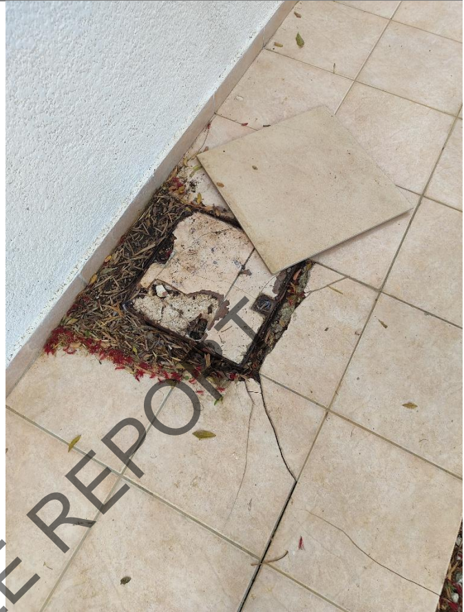
P2: Damage and deterioration noted to the external sewerage inspection chamber cover and surrounding tiled finishes, including cracked/broken cover sections and localized displacement/damage to adjacent tiles
