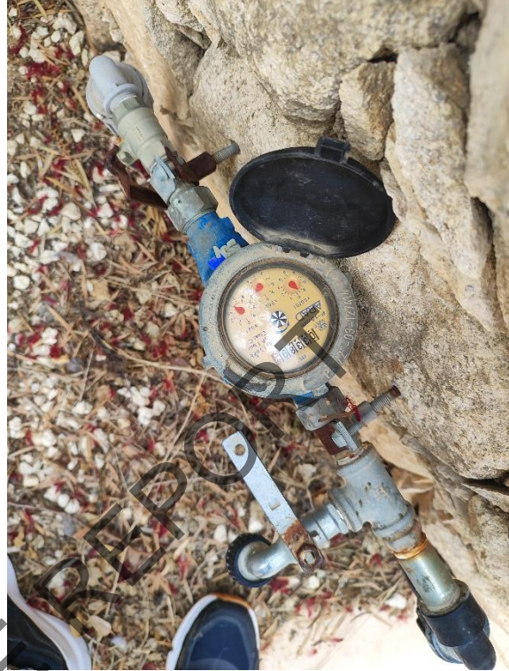
P2: Water meter of the property.
