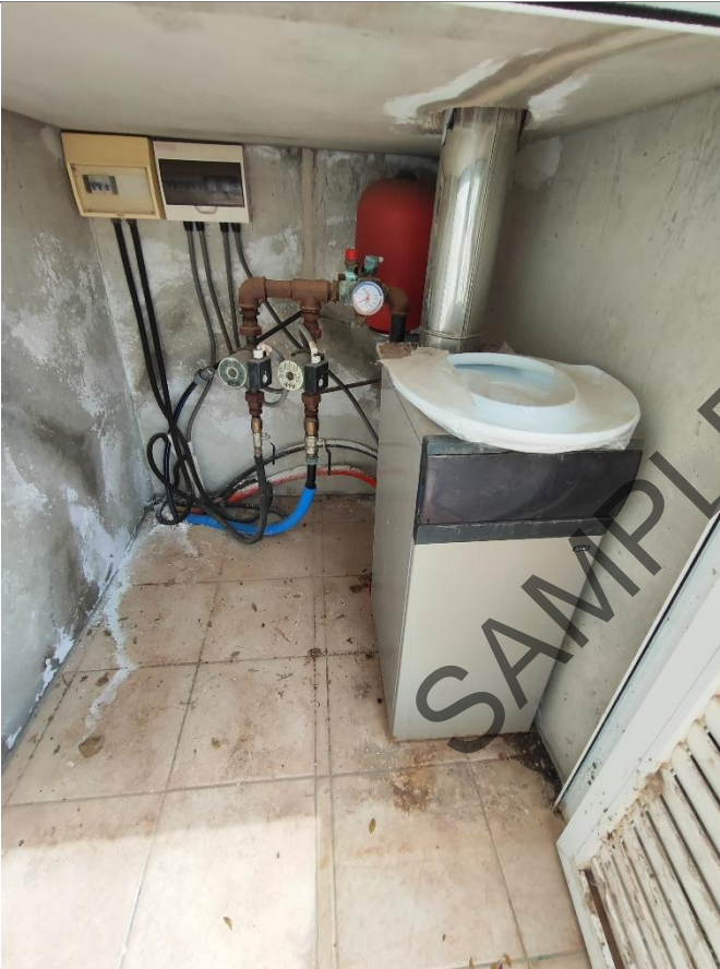
P1: Localized dampness, moisture staining, and deterioration to wall finishes were noted within the mechanical/plant room area, particularly at lower wall sections and around service penetrations.
