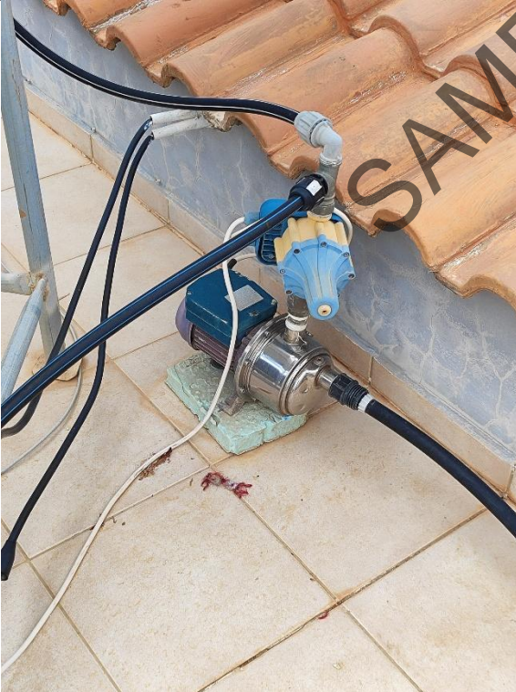
P3: Water pressure pump of the property.
