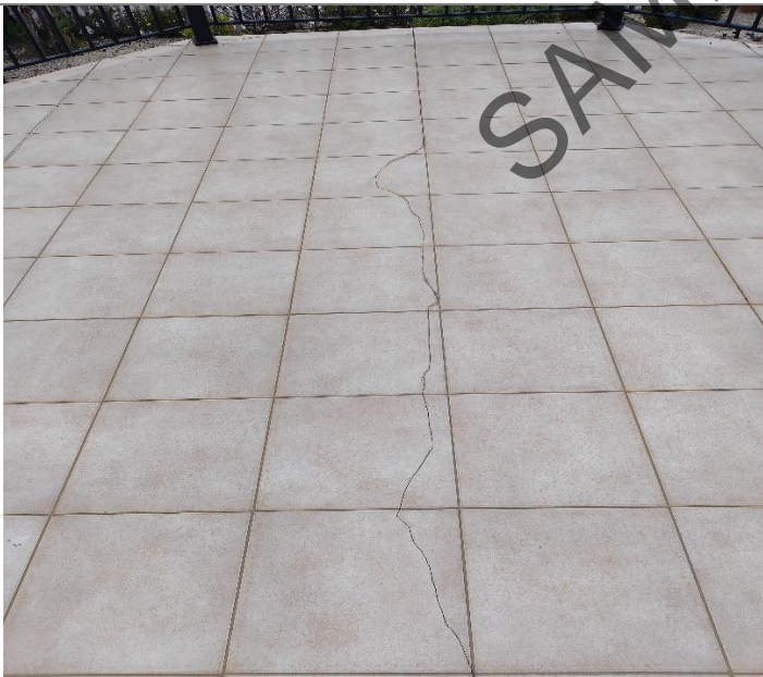
P5: Long continuous crack observed extending through multiple tiled sections across the roof garden tiled surface, including localized opening of grout joints.
