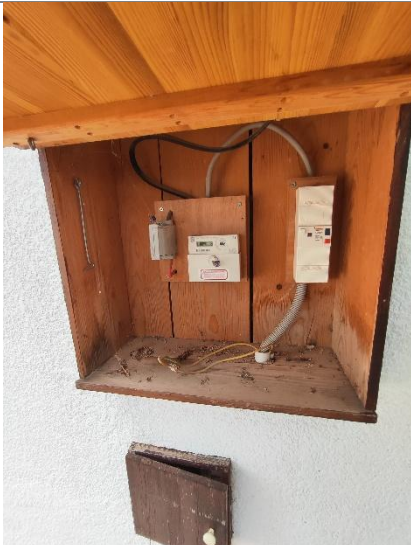
P1: The electrical meter of the property.
