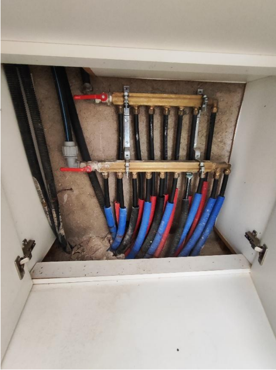
P1: Manifolds/distribution board
