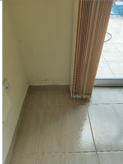
P2: Localized signs of possible rising damp/moisture-related deterioration noted to lower sections of the internal side of external perimeter walls
