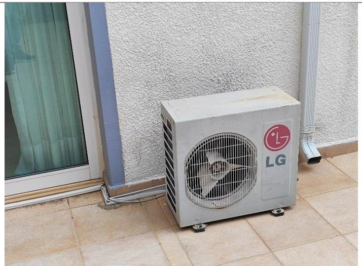
P2: Condenser/compressor units are installed externally
