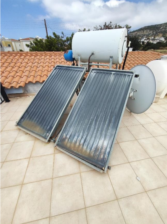
P1: Localized weathering, surface corrosion, and general aging noted to sections of the solar water heating installation and associated metal support frame/components at roof level consistent with prolonged external exposure conditions.
