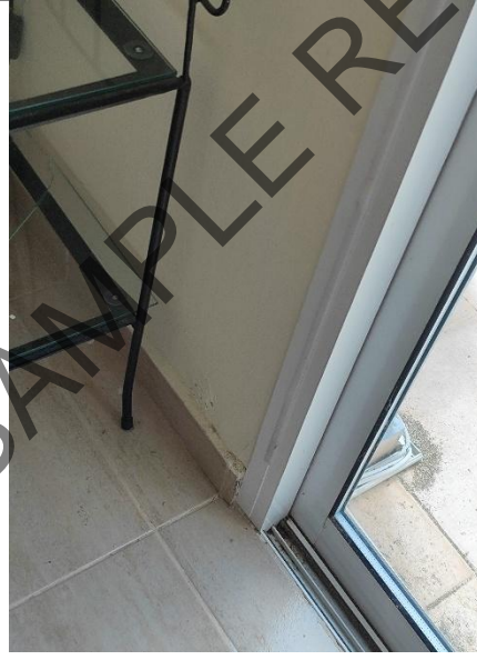
P5: Localized signs of possible rising damp/moisture-related deterioration noted to lower sections of the internal side of external perimeter walls
