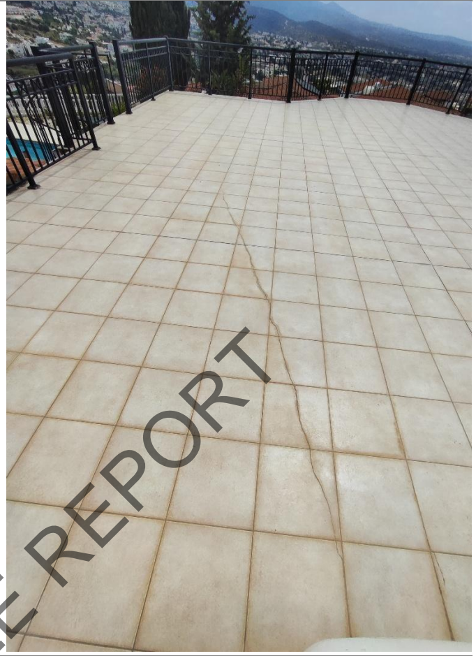
P4: Long continuous crack observed extending through multiple tiled sections across the roof garden tiled surface, including localized opening of grout joints.
