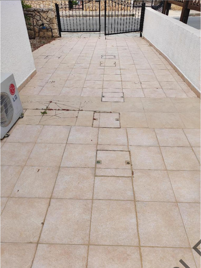
P1: Sewerage manholes around the property.
