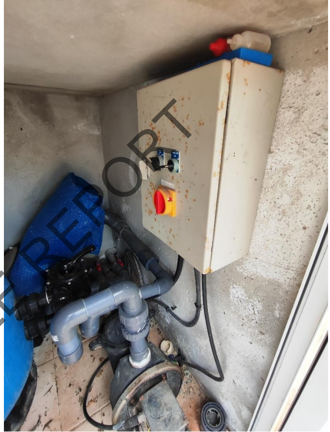
P2: Minor corrosion and weathering were also noted to sections of the electrical control cabinet and associated components.
